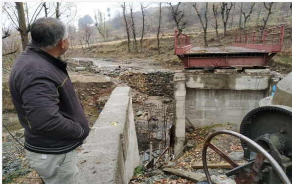
Construction of 1x10 mtrs span steel decked bridge on Gogaldara Nallah at Shuplin Gujjarbasti Sitaharam
