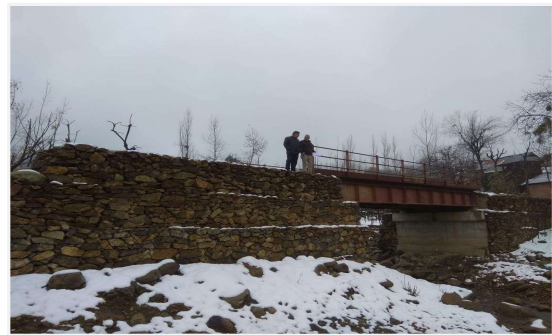
Construction of 1x12 mtrs span steel decked bridge on Wani Nallah at brass Gujjarbasti
