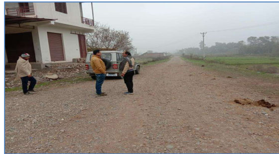
Constt of Road from border road Sc mohalla to Gujjar Basti Khandwal Pyt. Korepunnu
